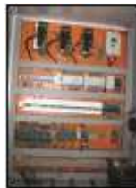
Control Panel For Grinding Machine (PLC)
