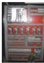
Control Panel For 12 Axis Press Break Machine
